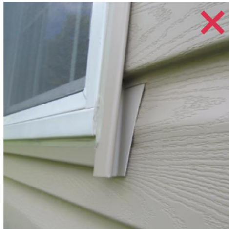
Figure 3: J-channel siding trim at the edge of an off-shelf clapboard cladding system prohibited. Proper trim required.
